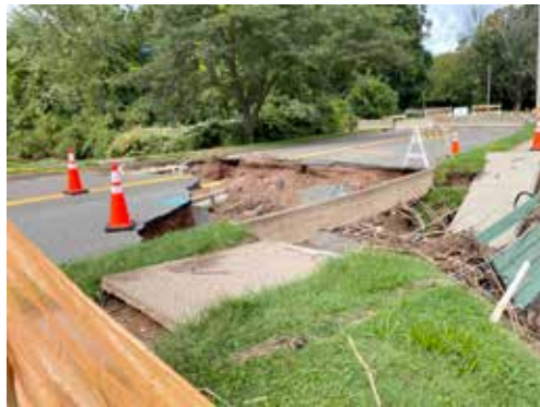
Severe rainstorm road washout, Town of Manchester
